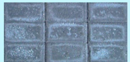
The effects of efflorescence on concrete blocks
